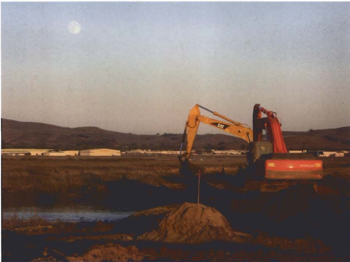
Figure 3. Completing construction of the NUB as Ponds 9 and 10 were opened to tidal action. Photo Courtesy of Ducks Unlimited, October 13, 2008.
