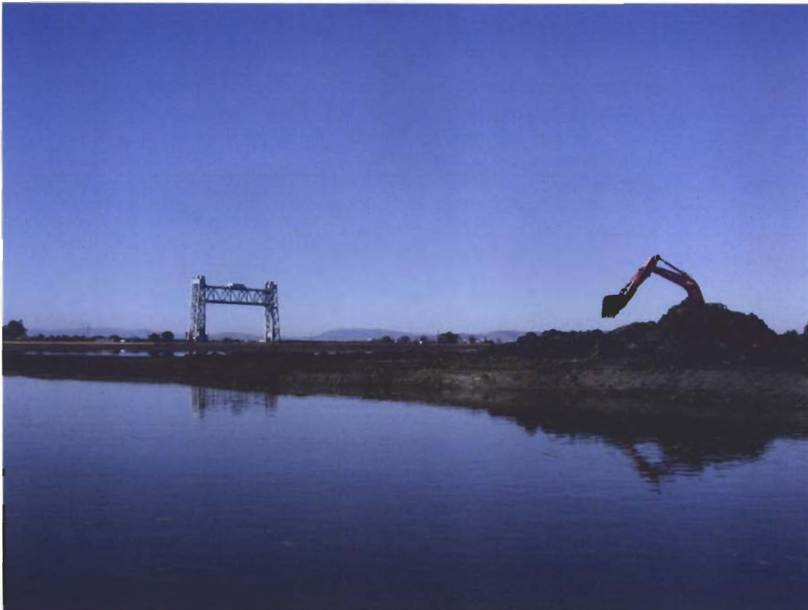
Figure 6. Levee lowering continues once the NUB was completed. One and one half tidal cycles have occurred when this photo was taken. K. Taylor, October 14, 2008
